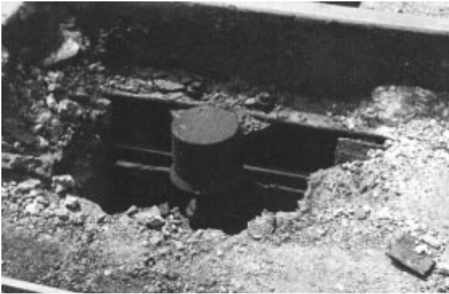
A hole in the existing roadway exposes an inverted metal can that shrouds the insulator. Two bolts hold the assembly to the lower flange of the running rail and one of the conductors can just be seen at the bottom.
